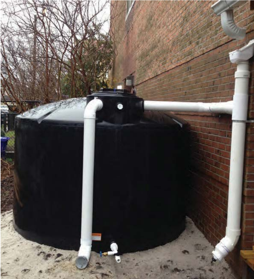
Figure 4.23. Example cistern application (photo: Marty Morganello).
